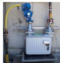
FCD installed on regulator
